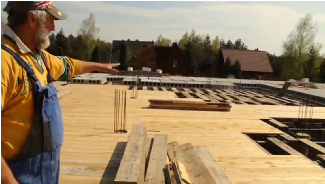
The unfinished timber support floor and no steel yet for the big slab
