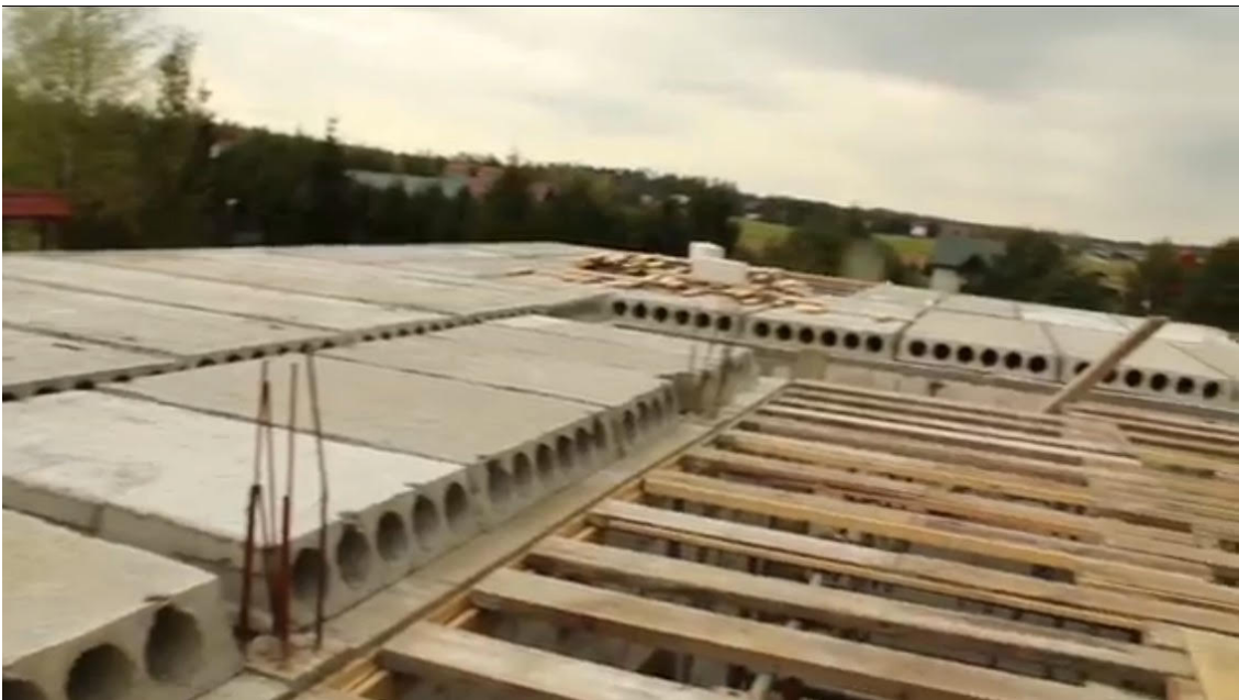
Pre-made slabs in place, a day the boys speak of, they will never forget – 7am to 9pm. Freezing – absolutely freezing and dangerous.
